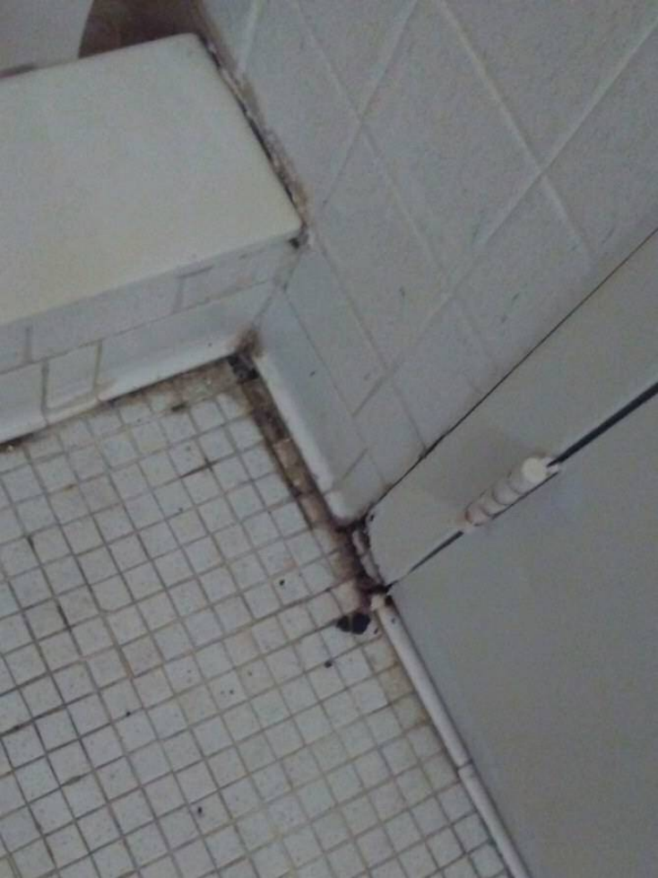
Mold in the shower at the group home housing a newborn and newly postpartum mother. Photo source: mother, before her phone was seized, who passed the photo on to the press and asked that it be published.
